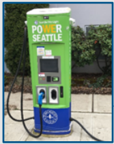
Seattle City Light DCFC charging station.
