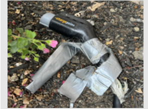
Frayed cables, open or cracked EV connectors, and broken insulation should be treated as hazards.
